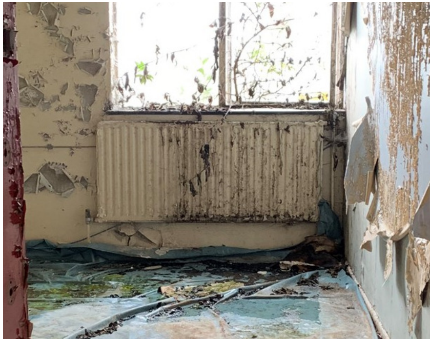
Plate 17: Steel panelled radiator
