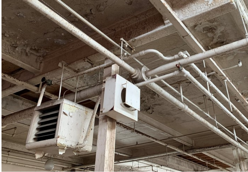
Plate 14: Space heating, PA system, sprinkler system and pipework
