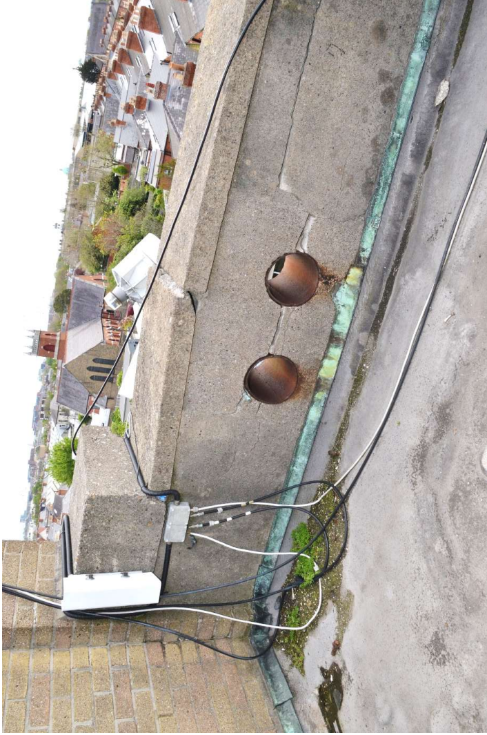
24. View of damaged parapet wall beside Room T8
