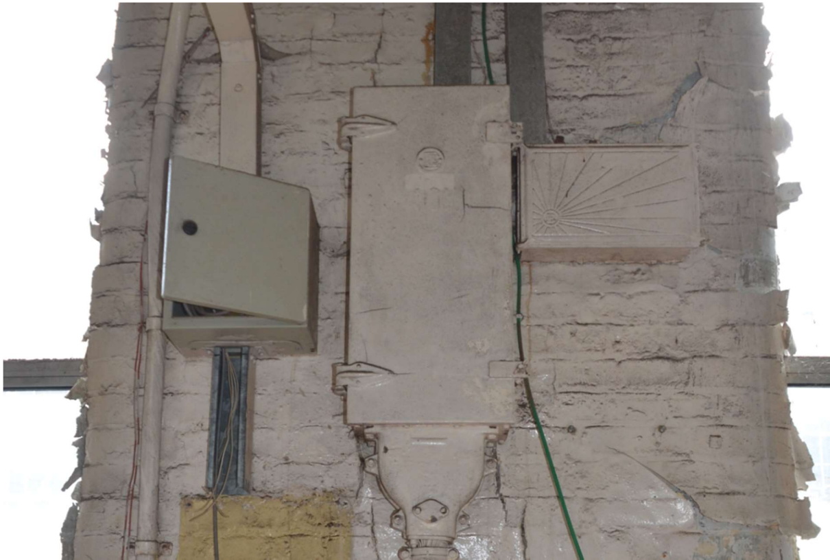
Figure 10: Decorative cast-metal cover to services box.
