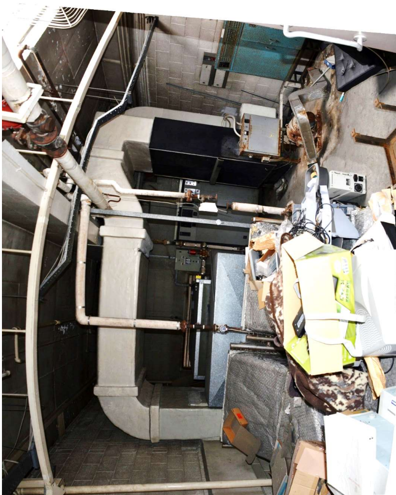
45. Service Room – First Floor Level
